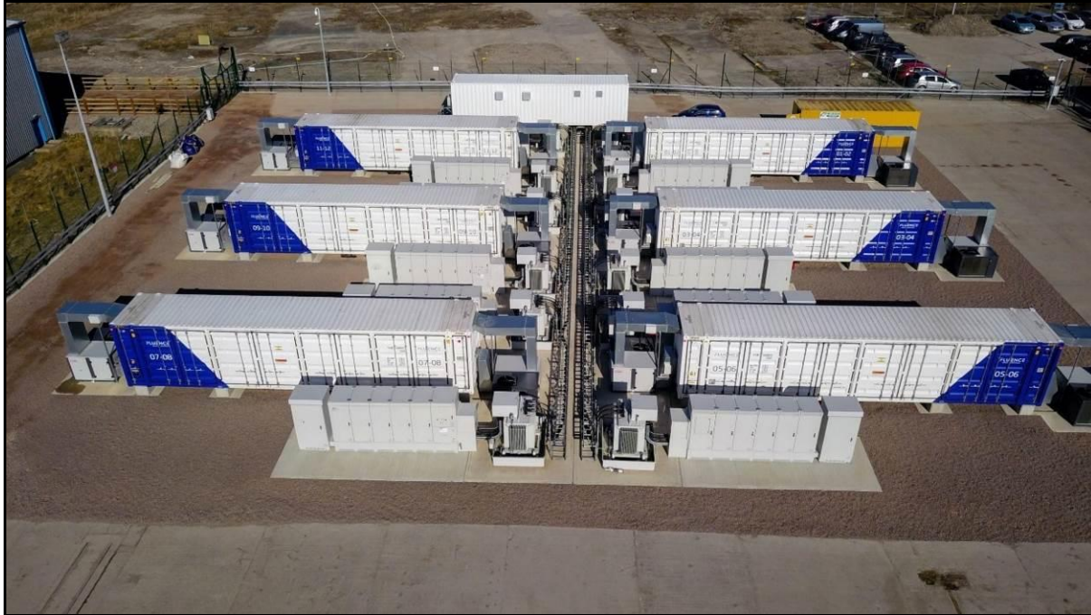
Photograph 1.2: Example of BESS located in storage containers
