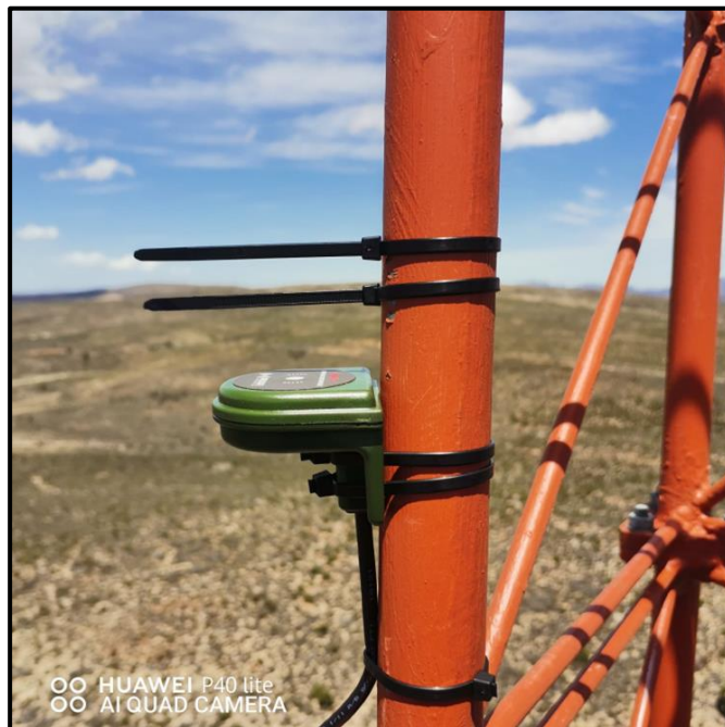
Figure 7: Example of mic on Met mast
