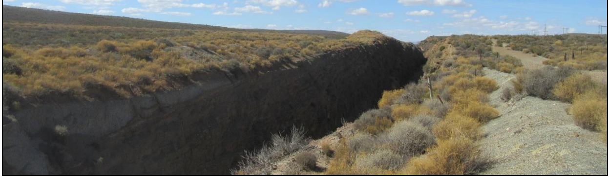
Photograph 3.5: Railway line cutting between Matroosberg siding and R318 to the west of the site
