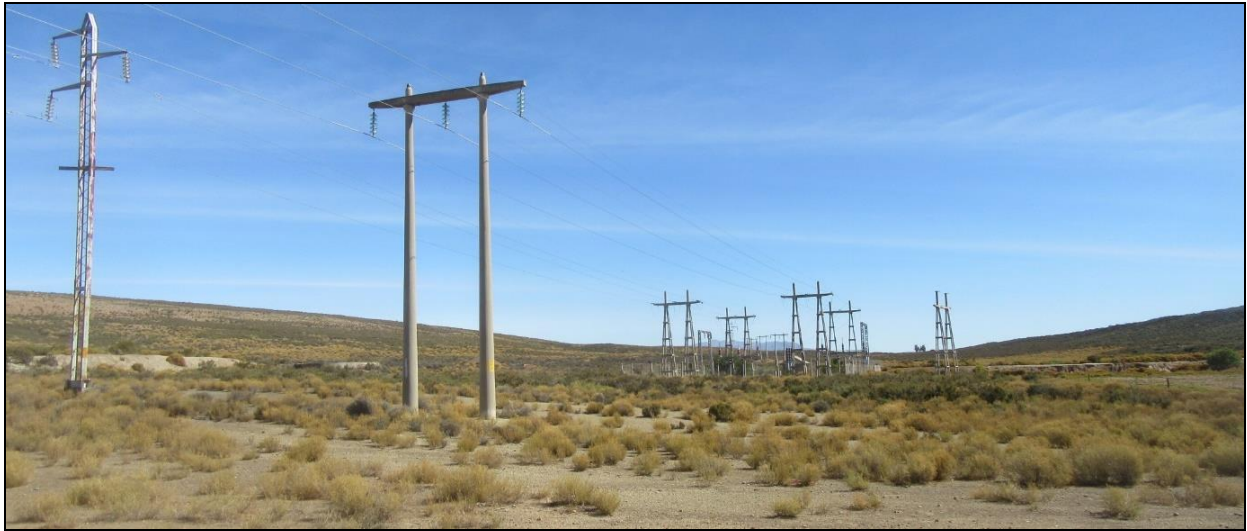
Photograph 3.6: Small substation near Matroosberg siding.
