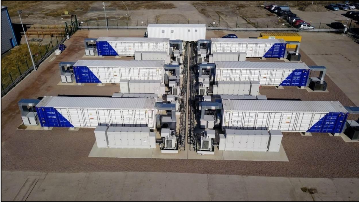
Photograph 1.2: Example of BESS located in storage containers
