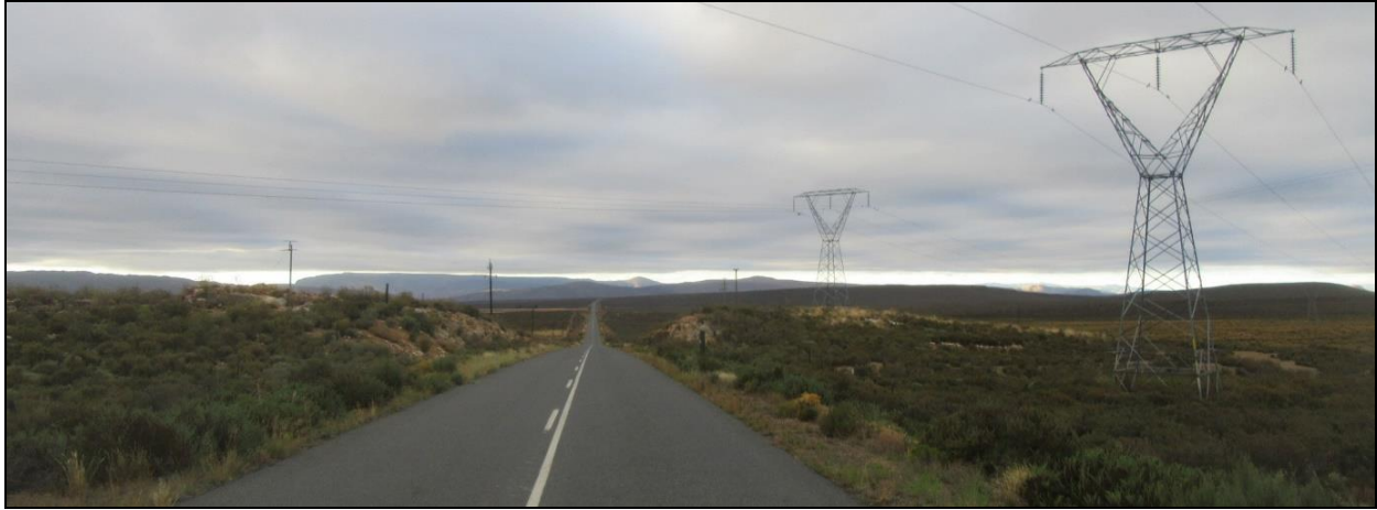
Photograph 3.7: 132 kV lines crossing the R318 on Stinkfontein Berg 147/RE (Hugo site)
