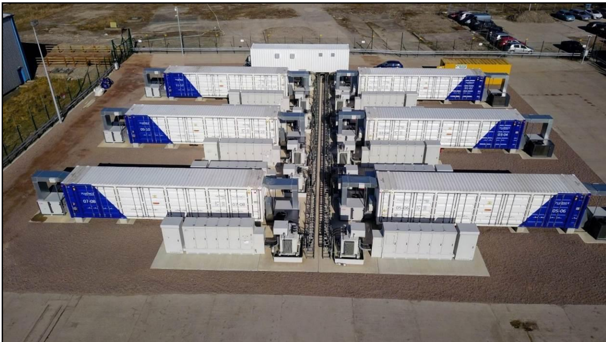
Photograph 1.2: Example of BESS located in storage containers
